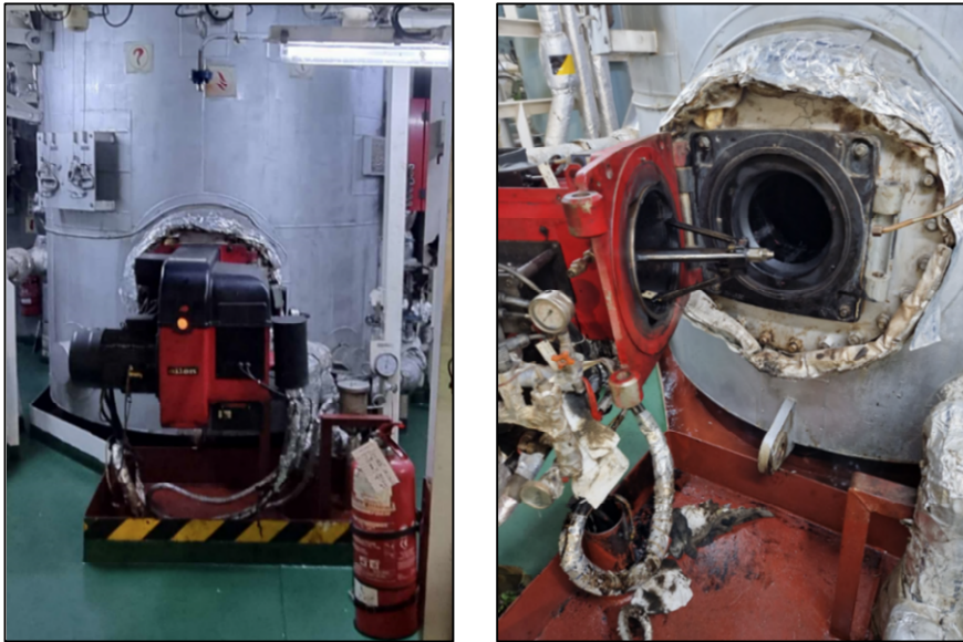
Auxiliary boiler with burner closed (left) and open during maintenance.
