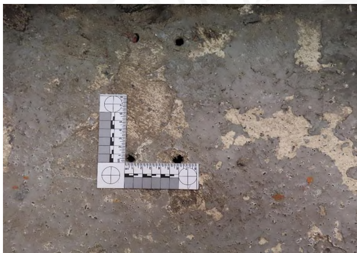
Islander II: Holes drilled in the bathroom floor to allow drainage of accumulated water
