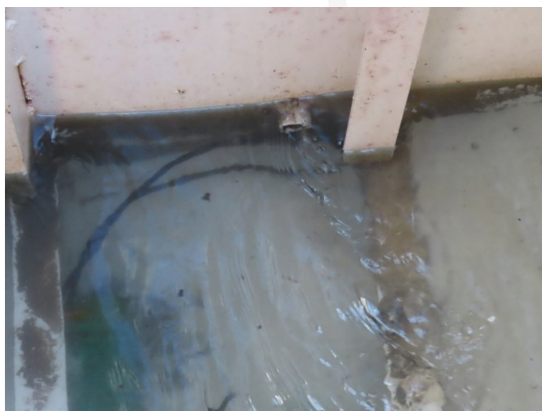
Islander III refloated hull: bulkhead penetrations allowing flow of water between compartments
