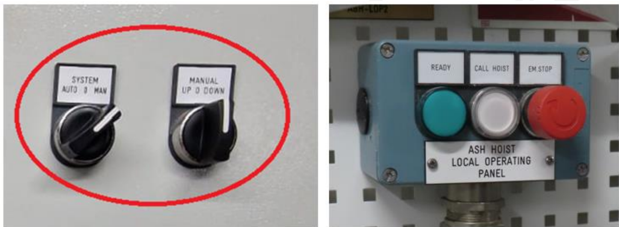
Figure 8. Main control box switch and smaller control box switch
