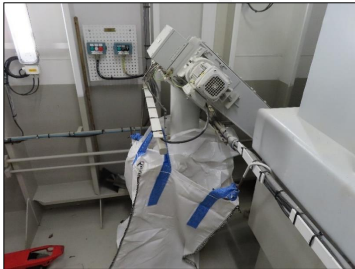
Figure 1. Incinerator ash discharge chute and bag
